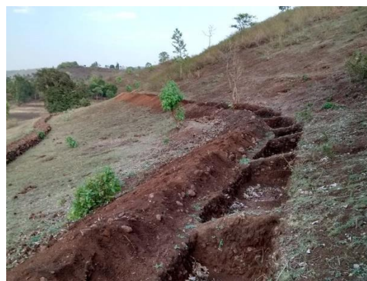
Figure 4. Water Absorption Trench.
